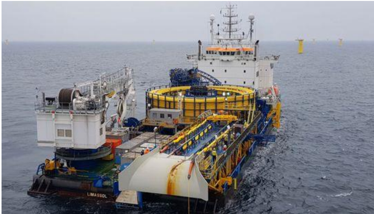
Figure 3.14: Example of inter-array cable installation at the EnBW Hohe See Offshore Wind Farm construction site in the German North Sea.
